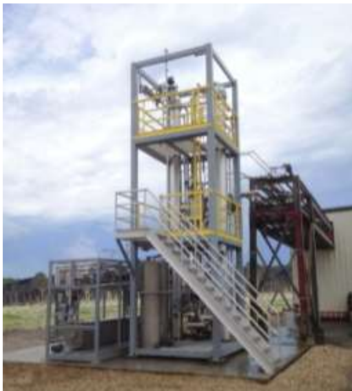
Distillation & dehydration modules installed at the University of Florida Stan Mayfield Biofuel Center
